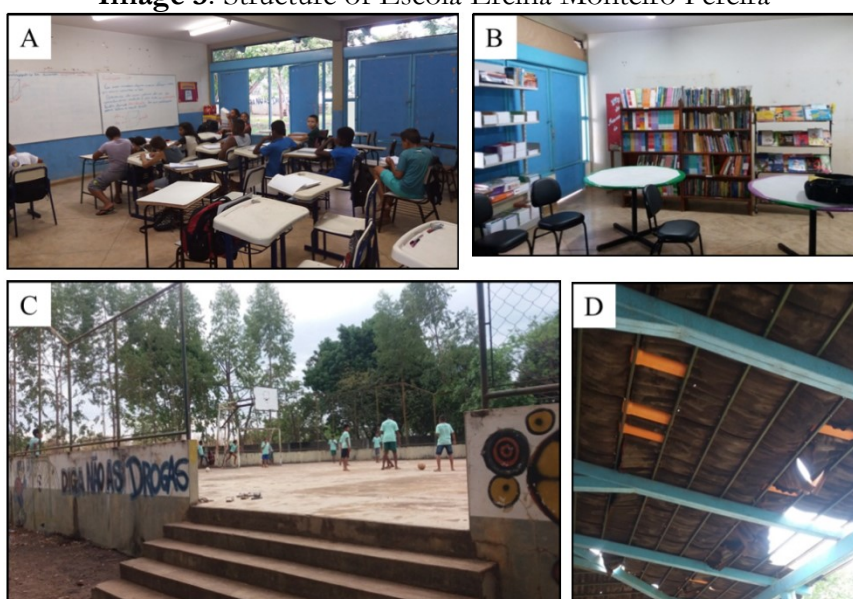
(A) Classroom; (B) Library; (C) Sports court; (D) Damaged roof.
